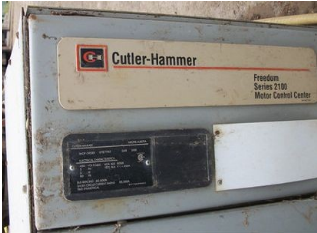
Cutler Hammer MCC Section. 480 Volt. 600 Amp Vertical and Horizontal Boss
