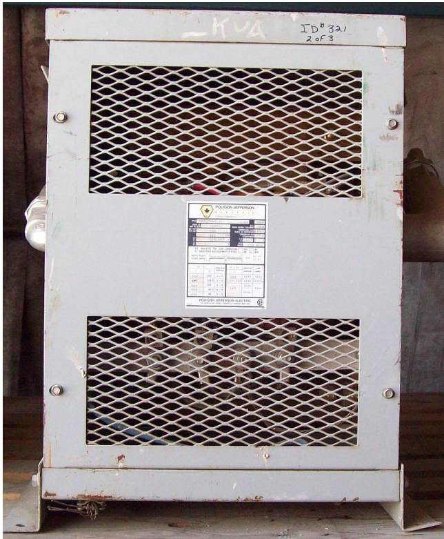
25 KVA 480 - 120/240 Single Phase Indoor Dry Polygon Transformer
