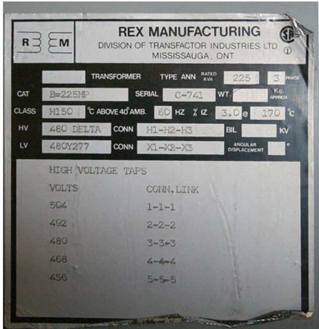
225 KVA 480 Delta - 480Y/277 Volt 3 Phase Indoor Dry Rex Manf. Transformer
