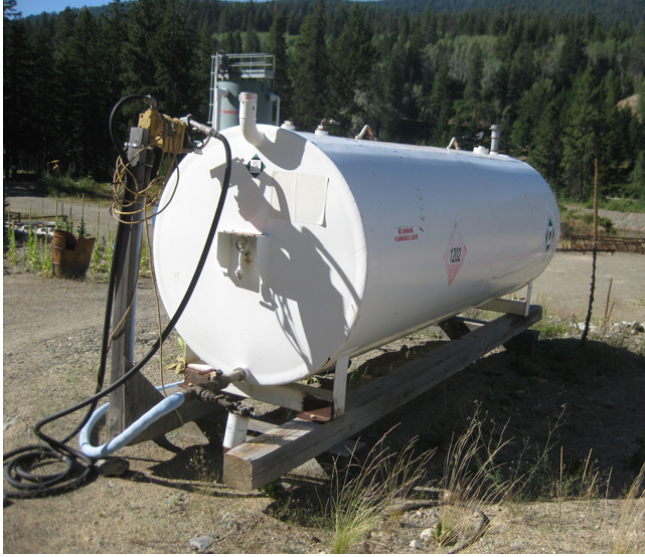
1000 Gallon Enviro Double Walled Fuel Tank.
