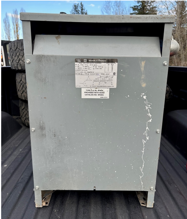
Square D 45kVA Multi Tap Transformer
