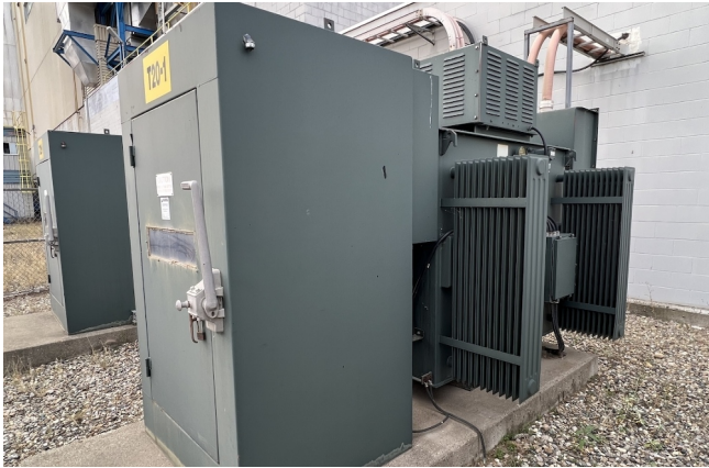
Ferranti-Packard 2000kVA Oil-Filled Transformer
