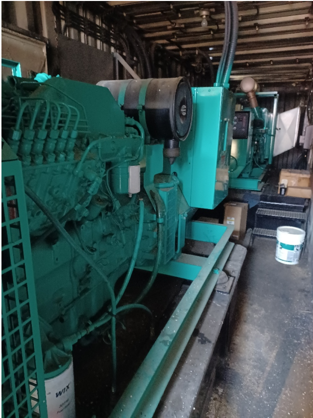
Dual 150kW Cummins Diesel Generators
