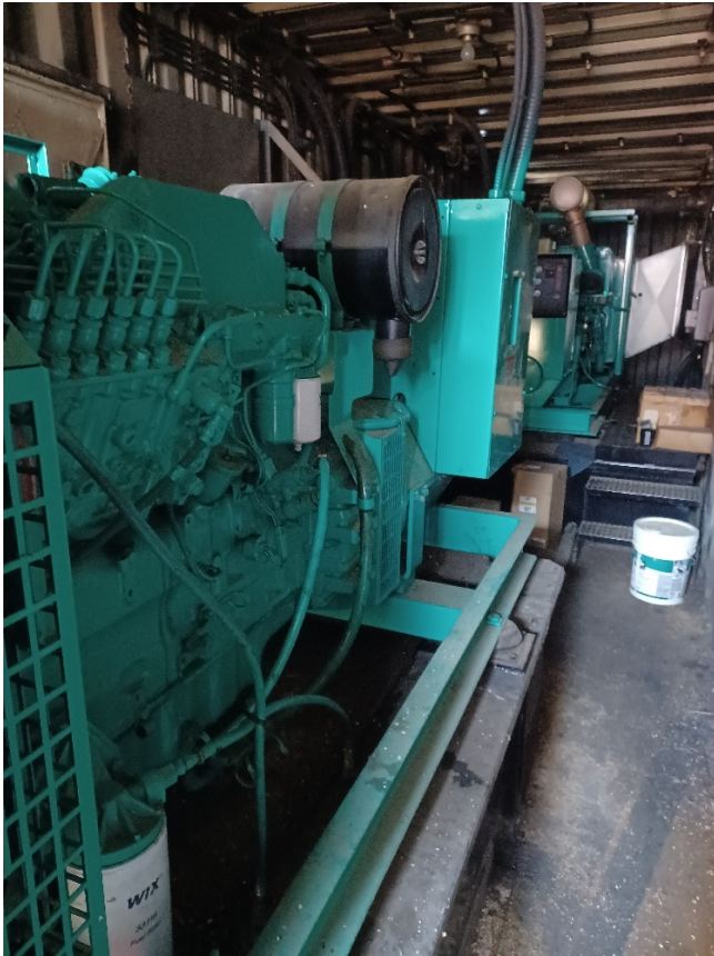
300kW Cummins Diesel Generator
