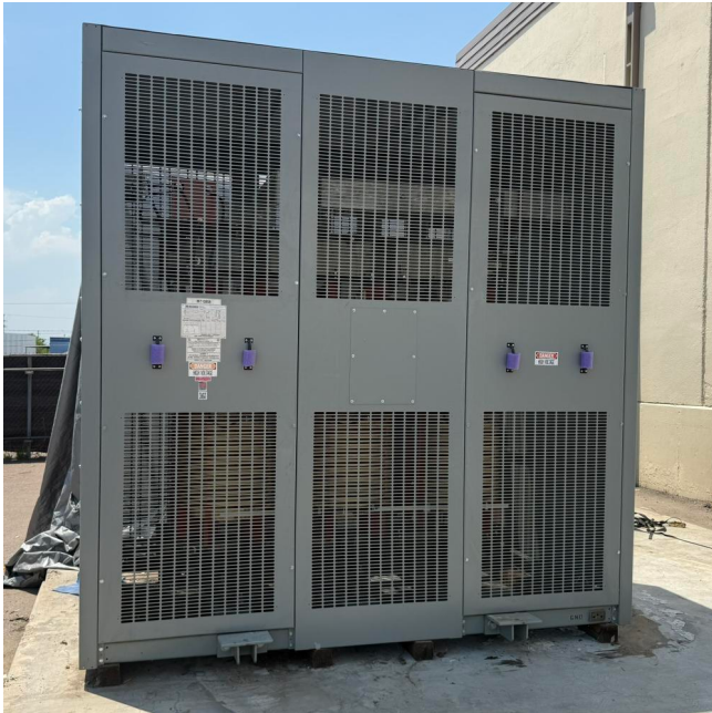
3000kVA Maddox Dry Type Transformer
