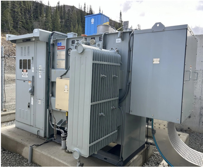
3000kVA Liquid-Filled Transformer
