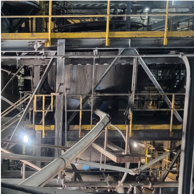
106in Dia. x 29.5ft Flotation Column Cell
