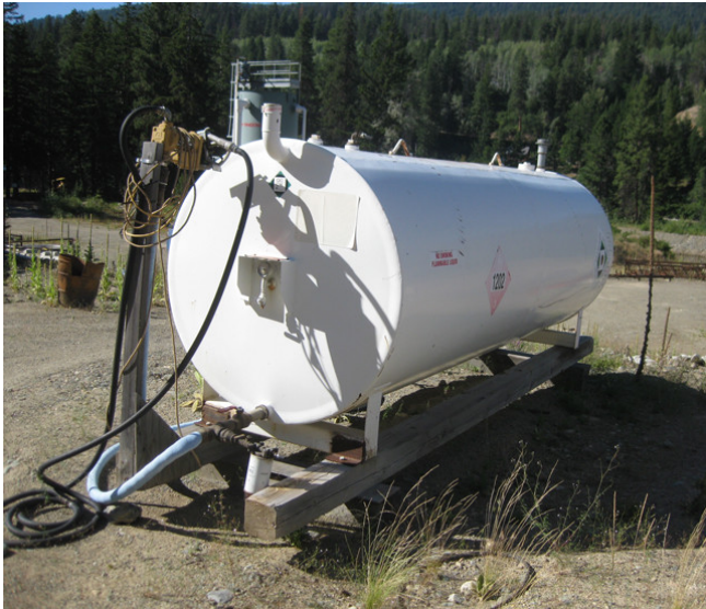
1000 Gallon Enviro Double Walled Fuel Tank.
