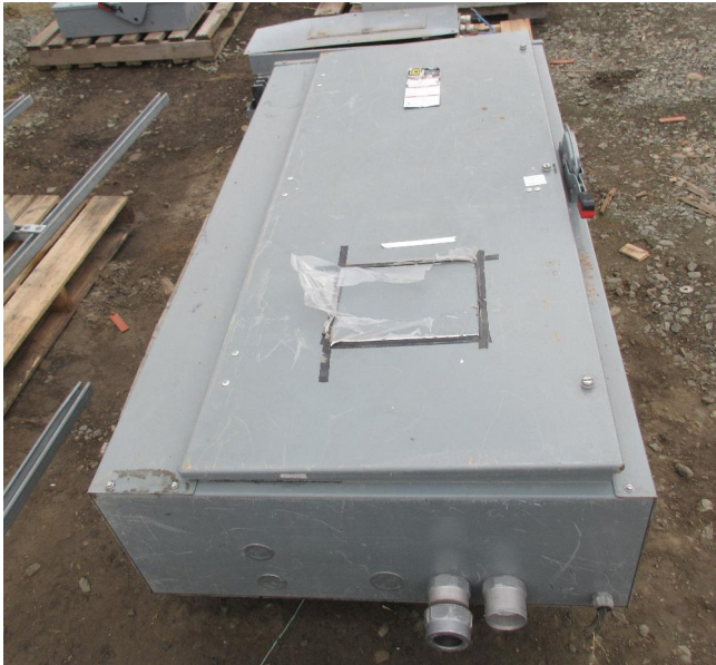
Square D 800 Amp Fusible Disconnect
